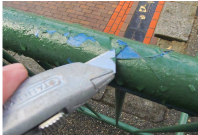
Photo 35 shows the condition of the coatings applied to the handrails at Centennial Station. An adhesion test was also conducted and indicated poor coating adhesion.
