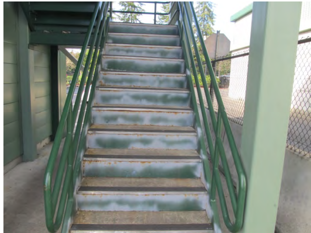
Photo 23 shows the rust that has formed on the edge of the steel.
