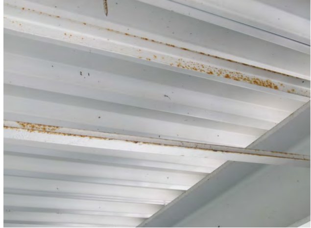
Photo 22 shows the rust that is present on the roof support truss work.
