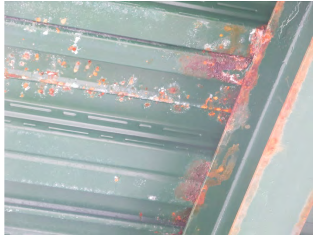
Photo 19 shows the spot rust that is present on the underside of the decking.
