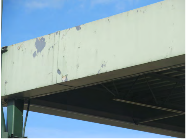
Photo 16 shows the delaminations on the fascia of the storage facility canopy.
