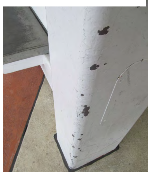
Photo 27 shows an example of the impact damage that is present on the posts at the transit center.
