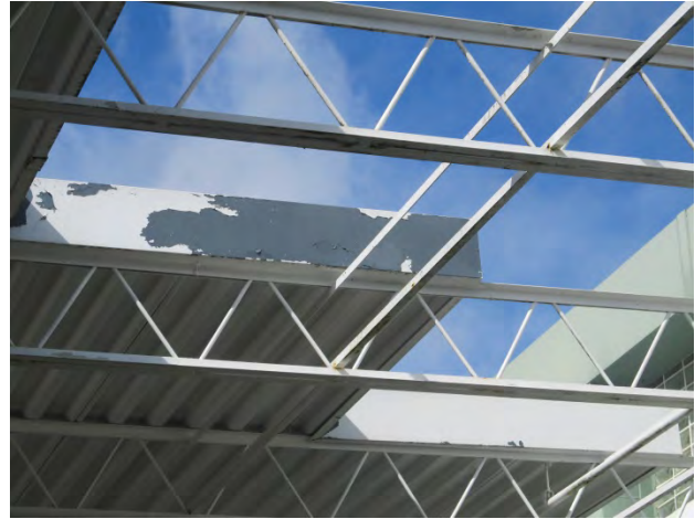
Photo 4 shows some of the delaminations that were found on the entrance canopy surfaces.
