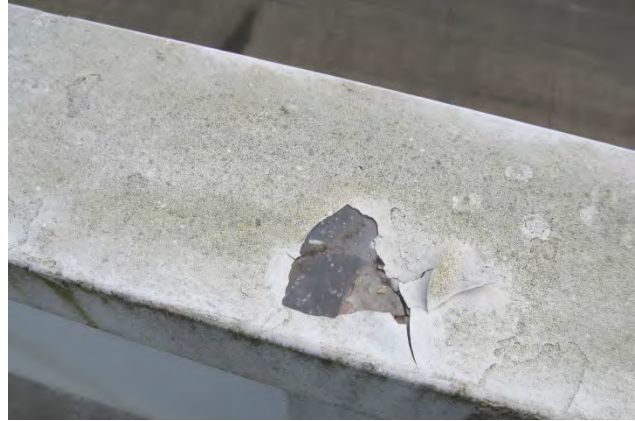
Photo 13 shows an example of the delaminated coatings on the parapet cap.
