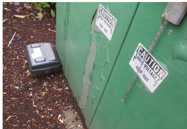
Photo 29 shows an example of the coatings on the transformers.
