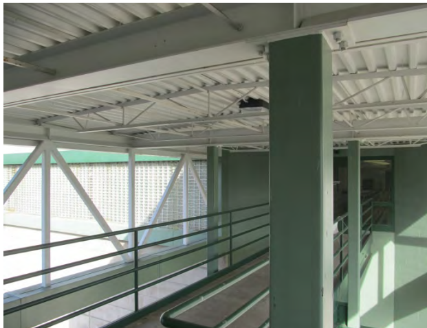
Photo 21 shows a general view of the bridge located at the western end of the Maintenance Facility.
