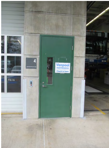
Photo 15 shows an example of the condition of the coating on the doors.
