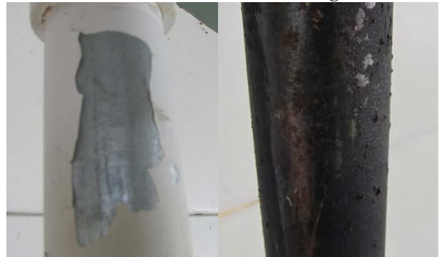
Photo 8 (left) shows a coating delamination on galvanized steel piping. The right photo shows a steel pipe with some delaminations. Rust was also present.
