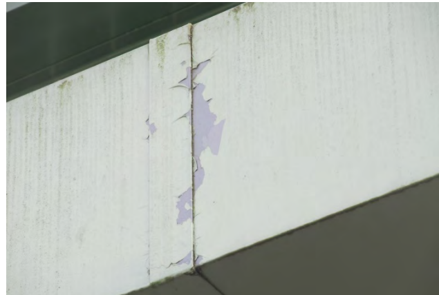
Photo 10 shows an example of the delaminations that were observed on the Maintenance Facility fascia and gutters
