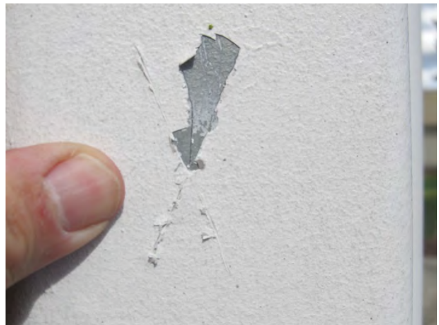
Photo 32 shows an example of the adhesion tests conducted, in this case, on the structural steel.
