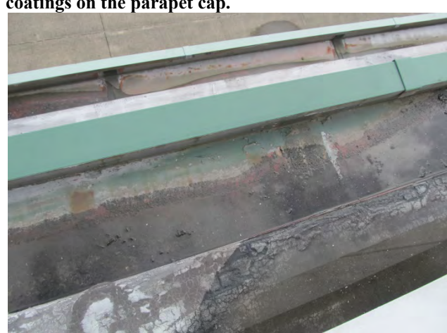
Photo 14 shows the condition of the box gutter interiors. Note the cracked thick elastomeric coating and the rust spots.
