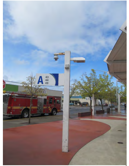
Photo 28 shows an example of one of the light standards. The impact damage at the lower portion of the standard is visible as well as the rust on the arm located at the top of the structure.
