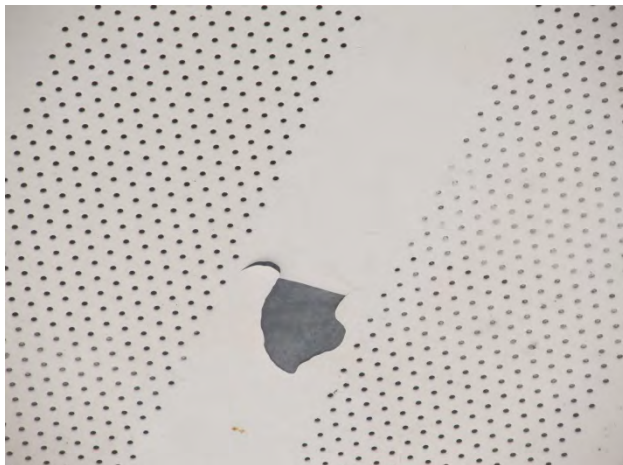
Photo 26 shows an example of one of the coating delaminations that are present on the roof decking.
