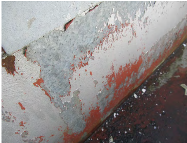
Photo 9 shows the condition of the gutter interior surfaces. Note the delamination from the galvanized steel surfaces.
