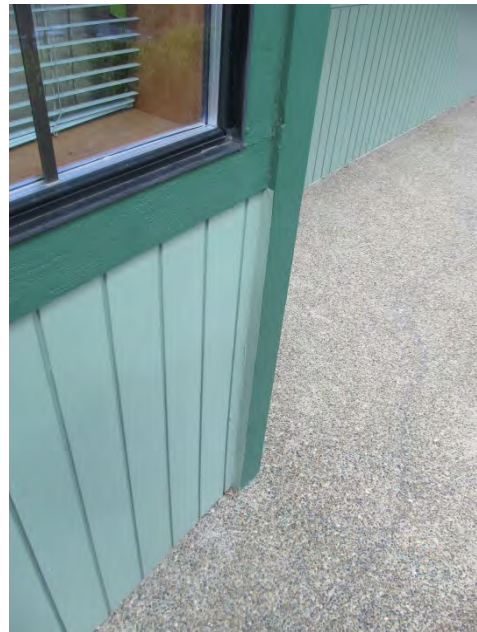
Photo 34 shows an example of the condition of the wood surfaces at Centennial Station.
