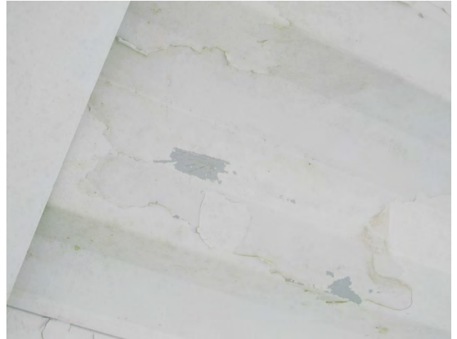
Photo 31 shows an example of the coating delaminations that were found on the decking at the Lacey Transit Center.
