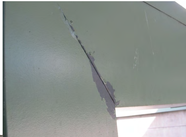
Photo 20 shows an example of one of the delaminations on the West Bridge fascia.
