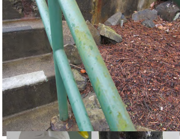
Photo 7 shows the typical condition of the railings at the east end of the administration building.
