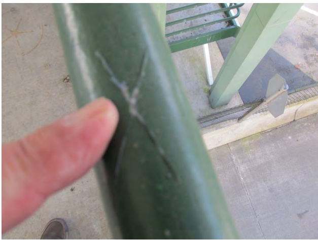
Photo 24 shows an adhesion test conducted on one of the railings. Adhesion is excellent on the railings.
